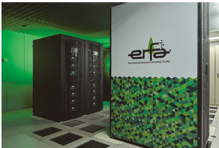
Fig. 1 NIES Environmental Research Computing Facility
