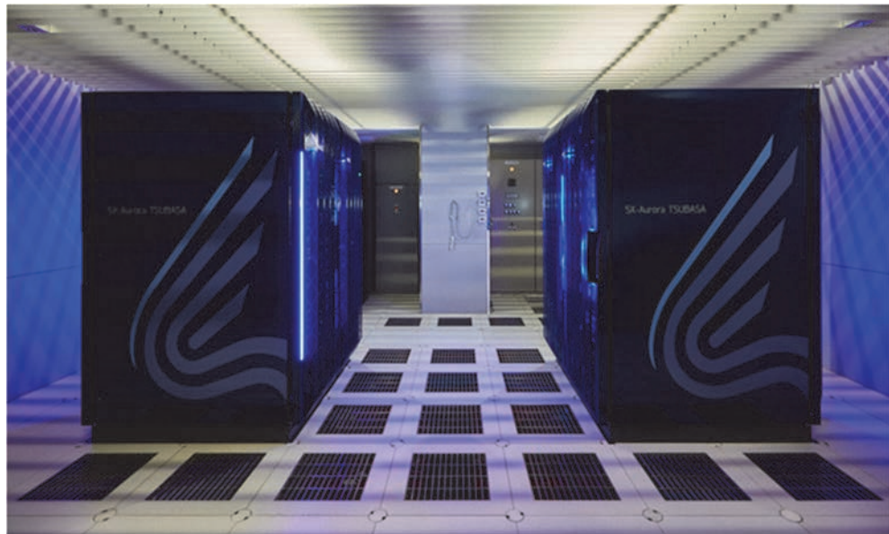
Fig. 1 The NEC SX-Aurora TSUBASA supercomputer.
